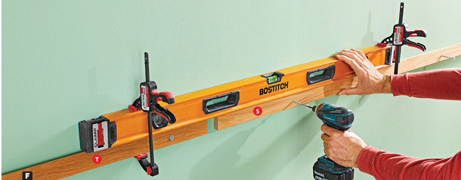
F Screw the cleats to the wall with 3½" screws. Drive screws into studs. Keep the tops of the three cleats level and even.
