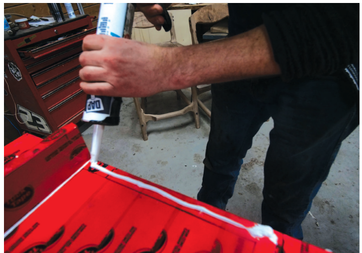
Seal the Joints – Because the joints all need to contain liquid epoxy, they need to be watertight. A healthy bead of caulking will help with this.
